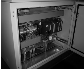
PLC in main control desk
