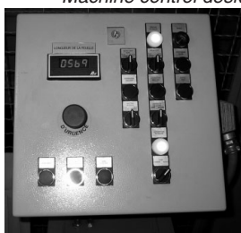
Machine control desk
